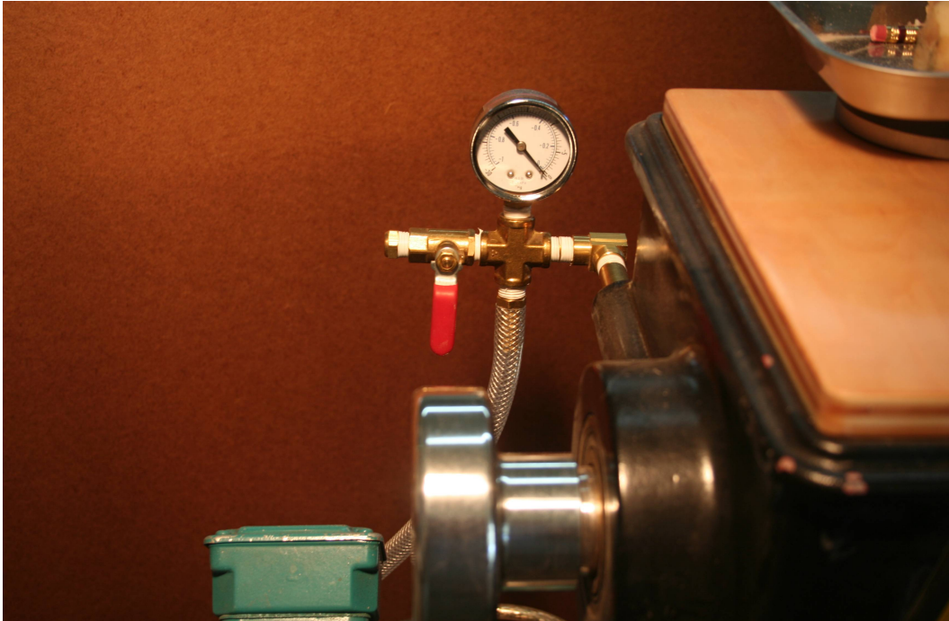
Factory Vacuum System -- Front View
